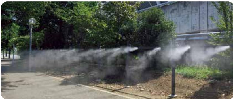
Dry mist cooling system at Tokyo Stadium
